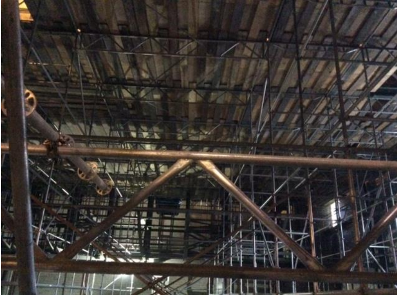
Partial view of Auditorium scaffold filling the space to allow for ceiling work
